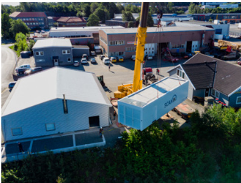
The installation of Canon's first relocatable MRI in Arendal in southern Norway.
